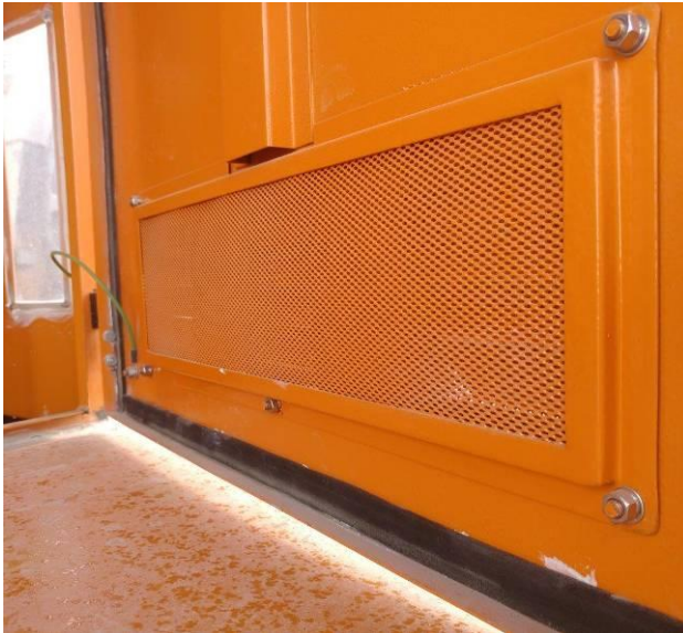
Door with the filter housing
